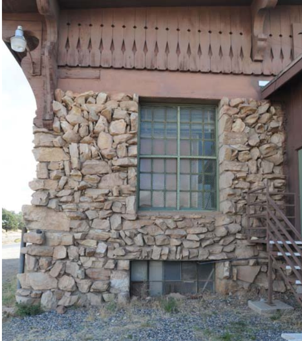
Existing northwest corner of Laundry Building showing grade against window glass
